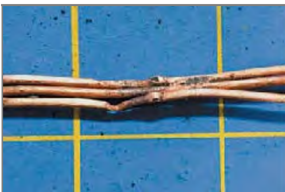
Figure 6.6.2.1(i) Copper conductors heated by fire and exhibiting a loss of surface characteristics and tool marks from the manufacturing process. This damage was created during a test burn.
