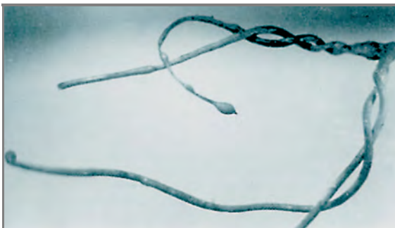
Figure 6.6.2.1(g) Stranded Copper Conductors Heated by Fire and Exhibiting the Loss of Strand Integrity of the Individual Strands.
