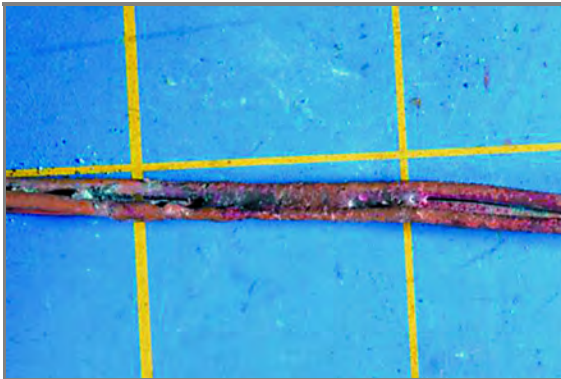
Figure 6.6.2.1(f) Copper Conductors Heated by Fire and Exhibiting Gradual Thinning of the Conductor.
