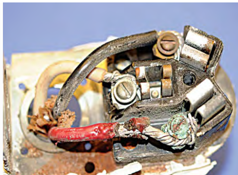
Figure 9.10.3.2(d) Overheated Connection on 120 V Duplex Outlet.
