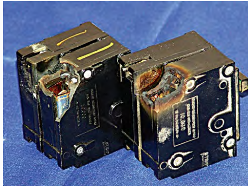
Figure 9.10.3.2(c) Overheated Connection on 240 V Dryer Outlet.
