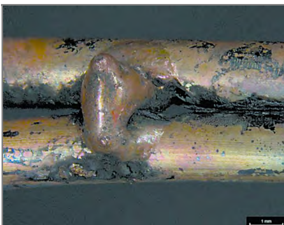
Figure 6.6.5.3.2(h) Nonmetallic Sheathed (Type NM) Cable Exhibiting Localized, Round Depressions/Notches in the Sides of the Conductors Created by an Electrical Arc. The ungrounded (i.e., hot) conductor is at the top of the image. This damage was created during a lab test.
