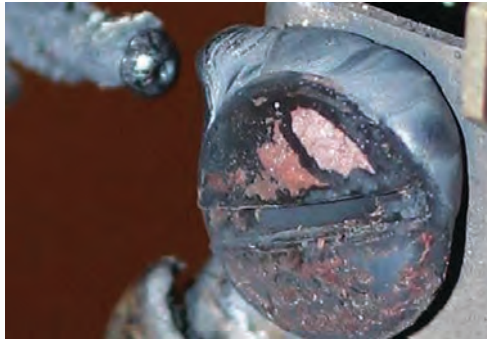
Figure 9.10.3.3(c) Enlarged Screw Head on Duplex Outlet Resulting from Severe High-Temperature Oxidation Adjacent to Glowing Connection.
