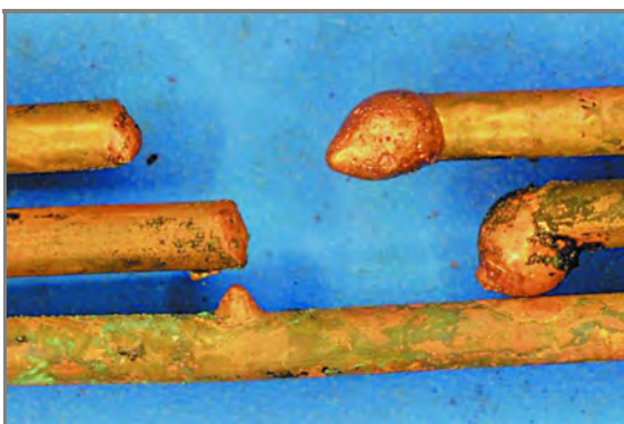
Figure 6.6.5.3.2(c) Nonmetallic Sheathed (Type NM) Cable Exhibiting Localized Contact Areas of Damage Created by an Electrical Arc. The ungrounded (i.e., hot) conductor is at the top of the image. This damage was created during a lab test.
