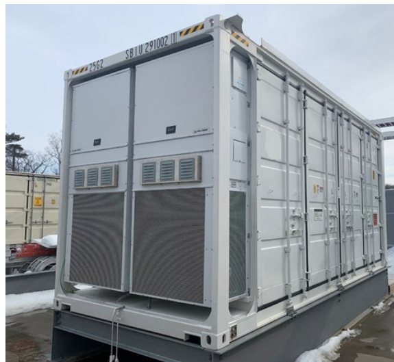
Figure 1 Battery Energy Storage Solution
