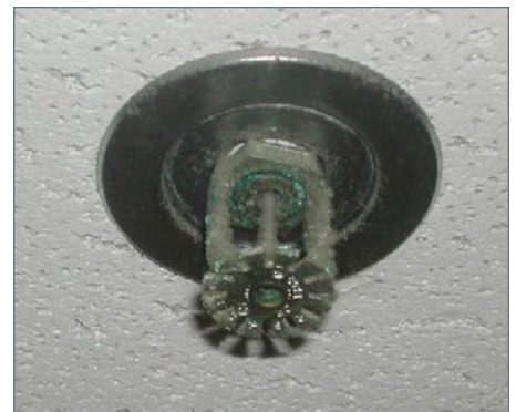
Sprinkler heads need to be maintained; accumulated dust or debris can act as an insulator and delay activation from the heat of a fire.
