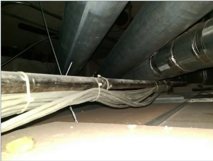
Cables should not be fastened to sprinkler pipes.
