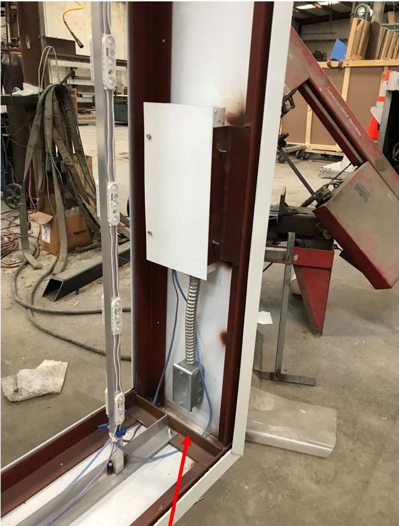
3 wiring method will terminate into a device box.
