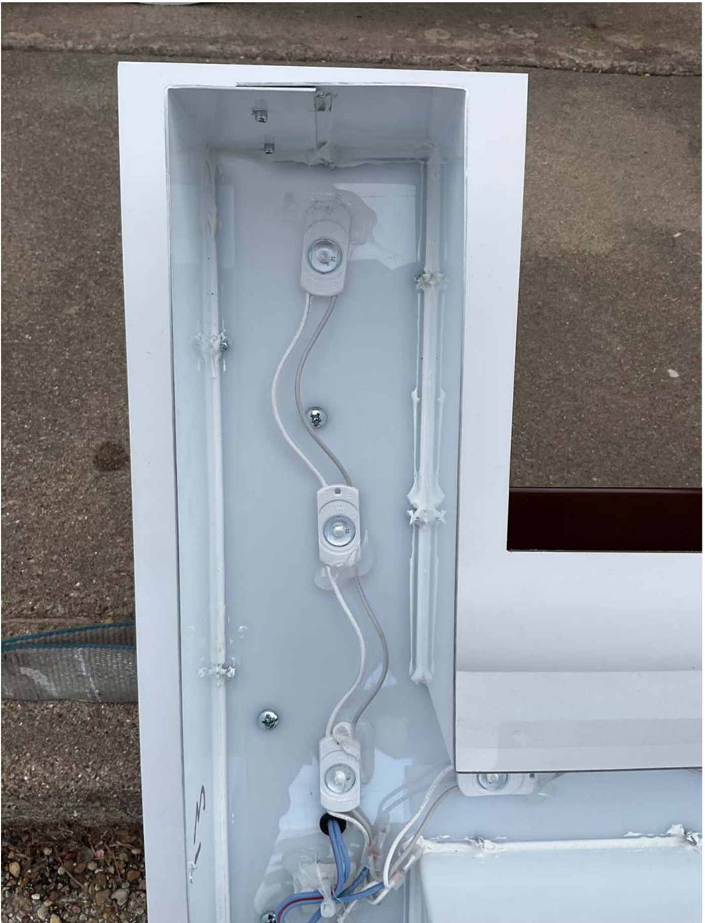
Halo rear illumination with Plexi glass illuminated face. Metal not bonded. 2 wire Class 2 cable installed.
