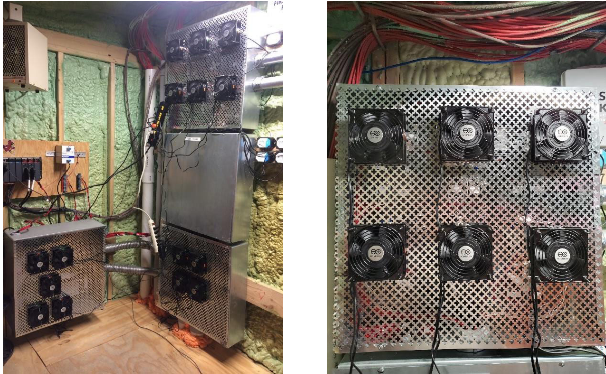
Figure 33. Cooling fans installed on the relays
