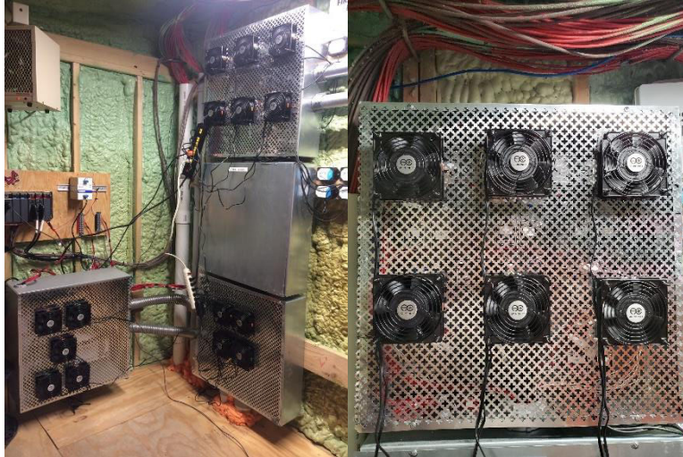
Figure B-1. Modification to address the overheating of relays
