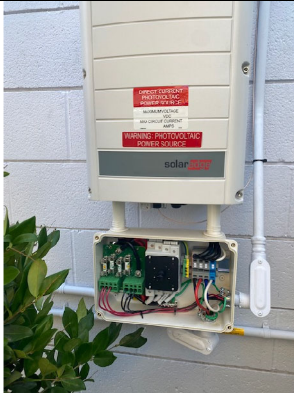
Photo 1 – Common Alternate Energy Installation
