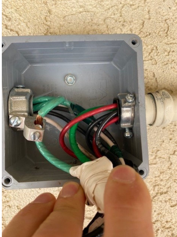
Photo 5 – Non-metallic Junction Box with EMT Raceway
