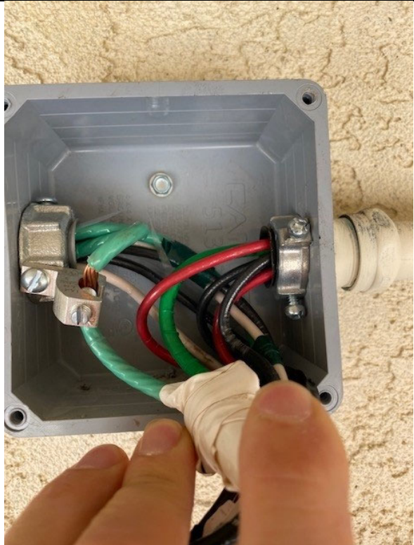
Photo 5 – Non-metallic Junction Box with EMT Raceway
