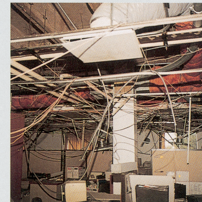
Suspended ceilings sustained damage in many installations, because sway wires were not used at all or installed improperly. Damage was extensive and very dangerous to people in the spaces below. Fortunately, the earthquake occurred when most offices were not occupied. Forces in this location were 0.2gV and 0.25gH.
