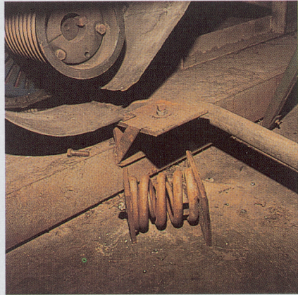
This close up of the spring shows that the attachment bolt broke allowing the spring to shift and fly free. (The spring was moved back for the photograph.) This would be a dangerous missile anywhere, but particularly in an equipment room with electrical devices. Proper snubbing would have controlled the situation.
