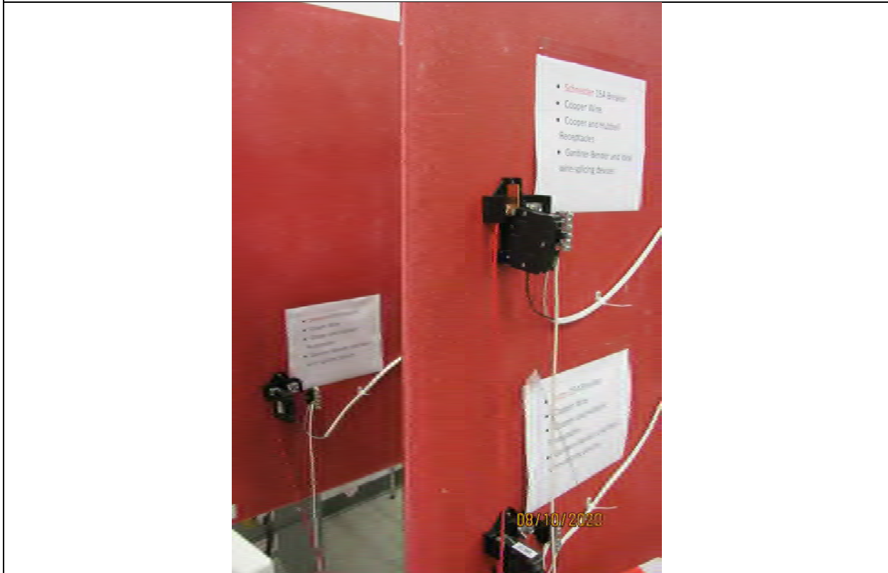
Photo 6 – Copper with Eaton and Hubbell Receptacles
