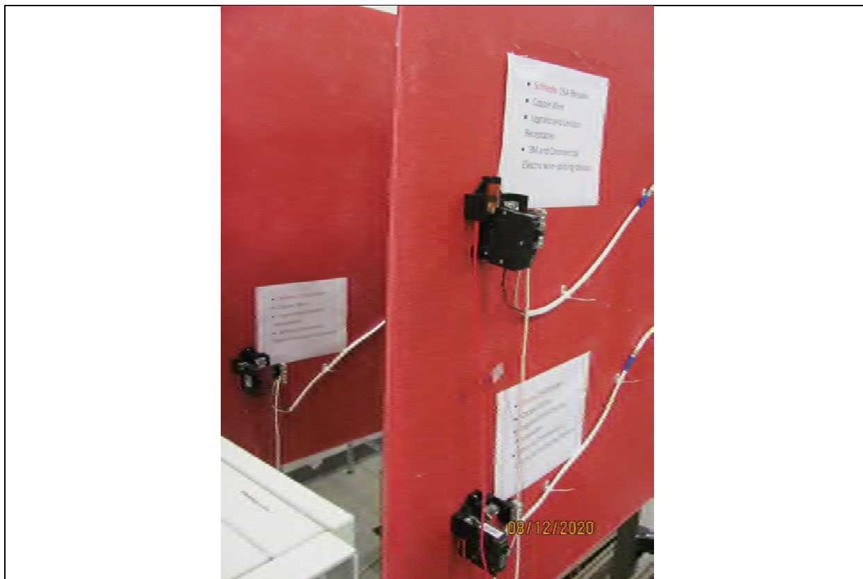
Photo 7 – Copper with Legrand and Leviton Receptacles
