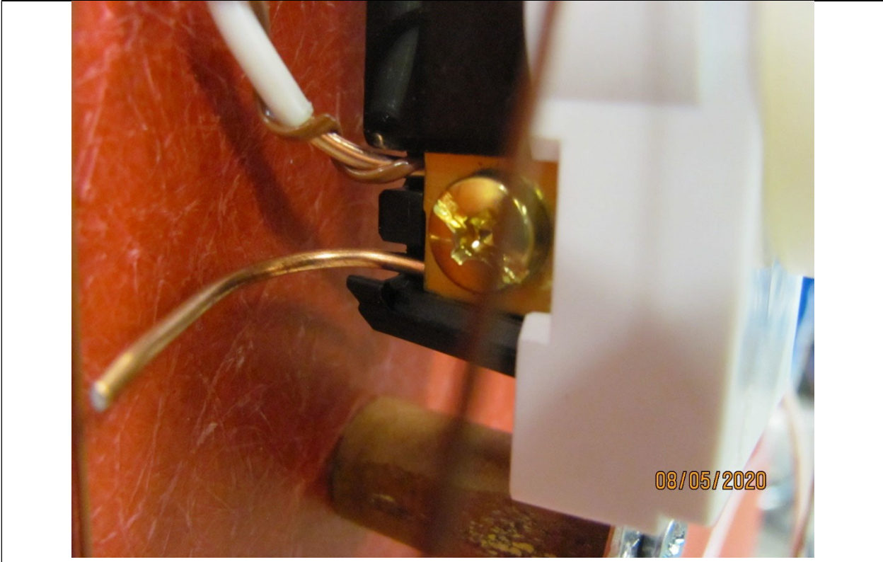
Photo 14 – Typical Installation of Receptacle Two Conductors Back Wired
