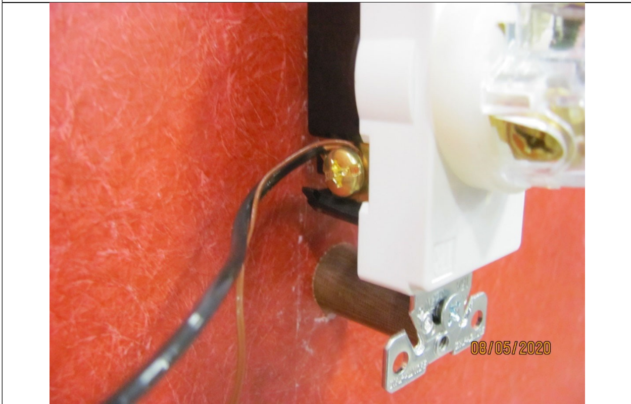
Photo 12 – Typical Installation of Receptacle using Wire Binding Screw
