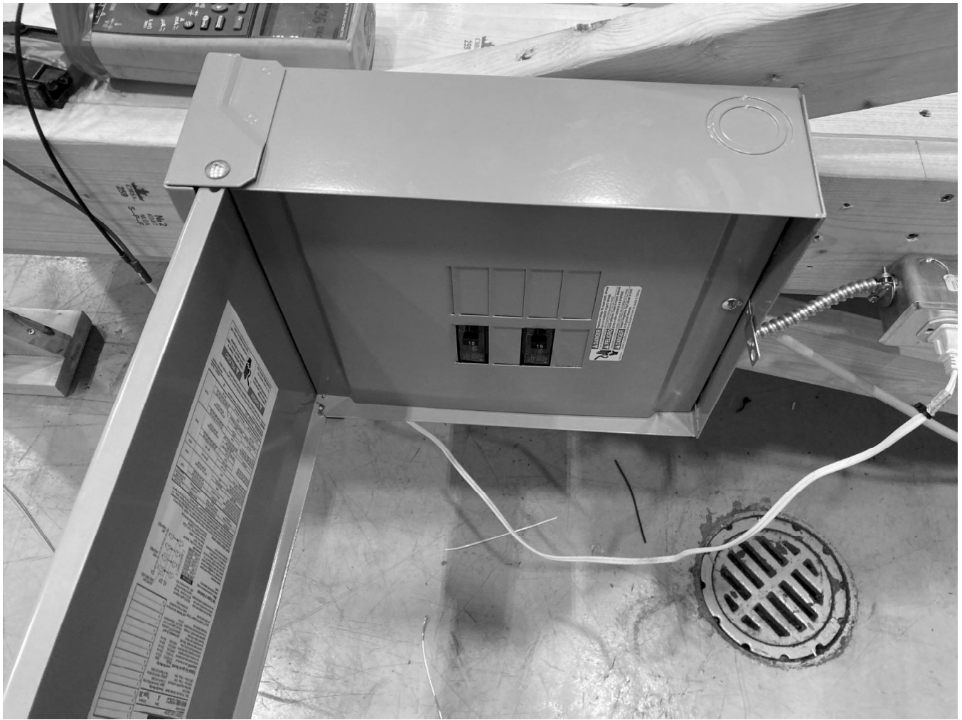
Figure B.7: Breaker Box
