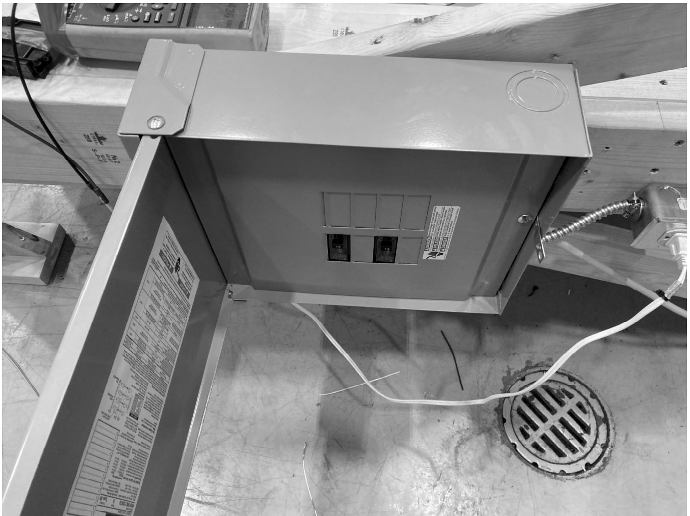
Figure B.7: Breaker Box
