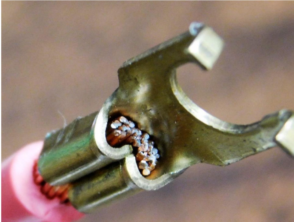
Appearance of Cord Terminals in August 2018
