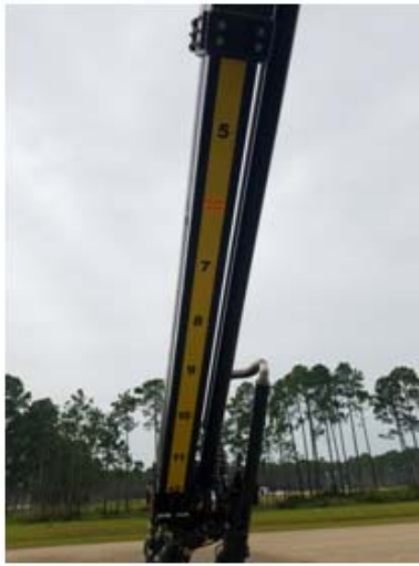
Photo of a simple marking system:
